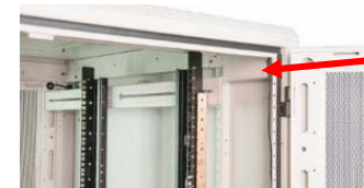
Concealed node & cable
