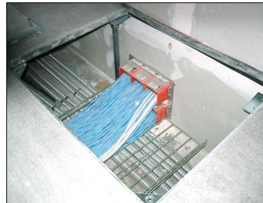
Below raised floor
