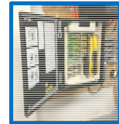
FDH Houses Splitters
