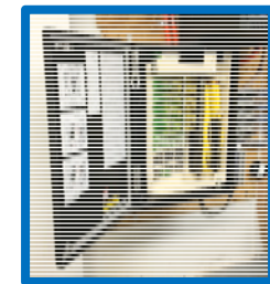
FDH Houses Splitters
