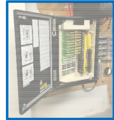
FDH Houses Splitters
