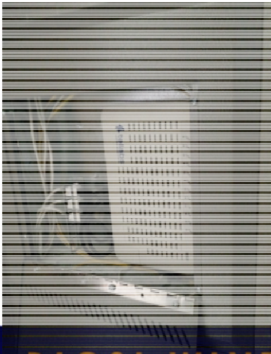
Secure Wall Box
