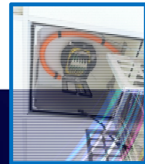
Consolidation Point Zone Cabling
