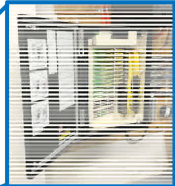
FDH Houses Splitters
